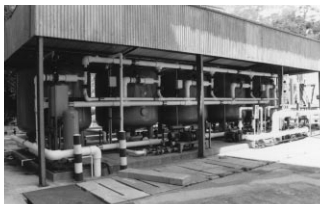
Figure 2 — Sand filters for brackish water pre-treatment
